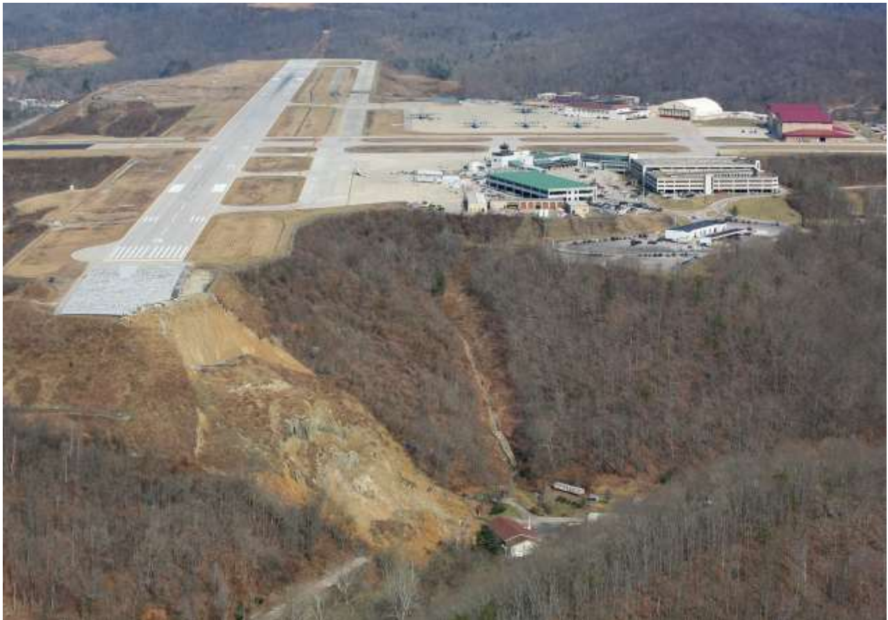
View of the collapsed Runway Safety Area on March 12, 2015
